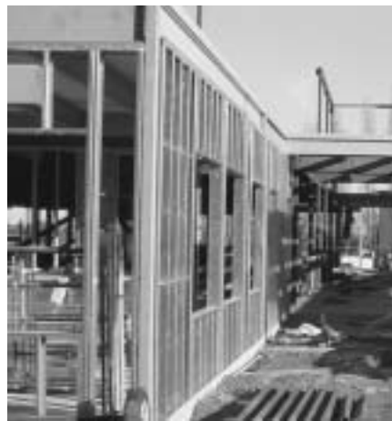
The superstructure of the West Shore Child, Youth and Family Centre begins to take shape in Colwood.
